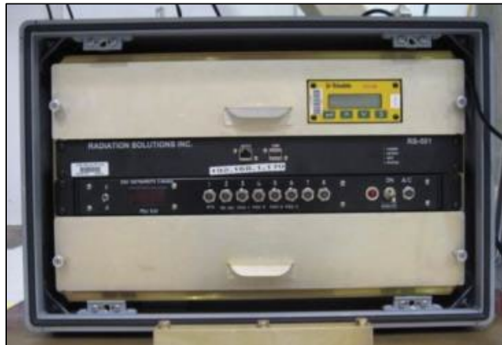
FIGURE 5. RS-501 AGGREGATOR CONSOLE WITH THE TRIMBLE GPS RECEIVER.
