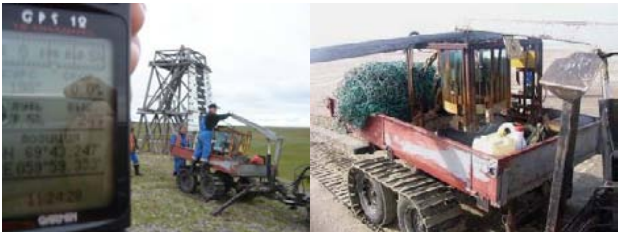
Fig. 3. RTG dismantling and its placing on a vehicle to deliver to the place where it is put on a pontoon. Each RTG dismantling shall be formalised in a deed signed by personnel involved in dismantling operations and approved by Head of operating organisation.
