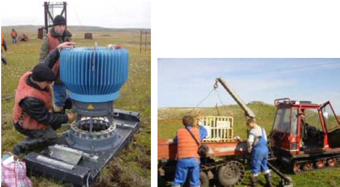
Fig.2. Preparation of RTG to dismantling. These operations are carried out by trained personnel of the operating organisation. A work permit is to be issued to execute this work.
